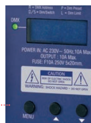
Panel de control.
